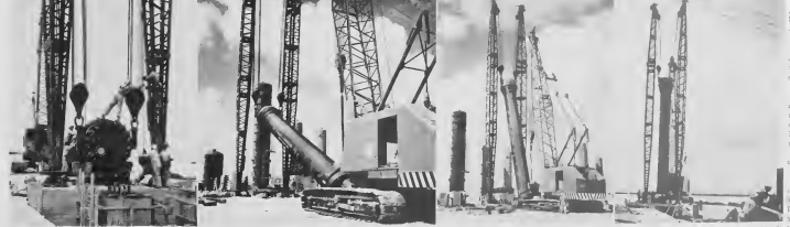
RIGGERS at the Antilles Chemical Company's construction site put strands of steel INSTALADOREN NA Antilles Chemical Company su lugar di construcion a pone cable di cable, gin poles and a 106-ton crane to the task of erecting the 120-ton ammonia converter waya di atal, balki di heru y un grua di 100 ton arriba e tarpa pa instala e convertidor di ammonia at Barcadera Juni 5. Workmen assemble over the top of the converter, left, and in succession of 120 ton ammonia converter, right, are used to pick up and swing the converter to its reinforced concrete foundation. den otro portretan e grua y homnan ta word usá pa lanta y move e convertidor pa su fundeshi di concreto reforzá cu lama.
